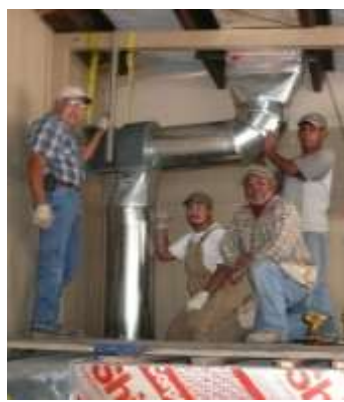
Our Hot Air Solar System Crew at work: Ernest, Javier, Felix, and Tommy. Team effort!
